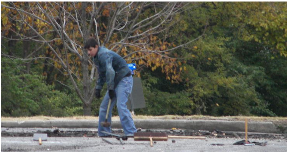
Milan Naster swinging the sledge hammer. Whew...how much more asphalt is left!??
